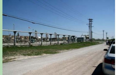
Compression station on Highway 303.
